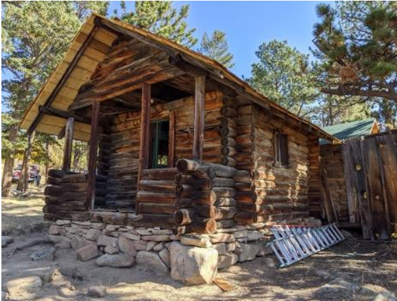
Main House and Laycook Homestead. Roof rehabilitated in summer 2020 by local volunteers.
